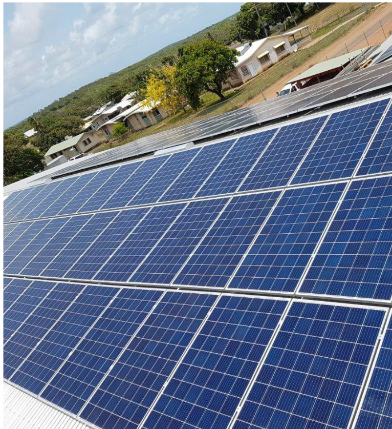
Figure 10: 750 solar panels have been installed in Lockhart River (below) to help reduce the community's energy bills.
