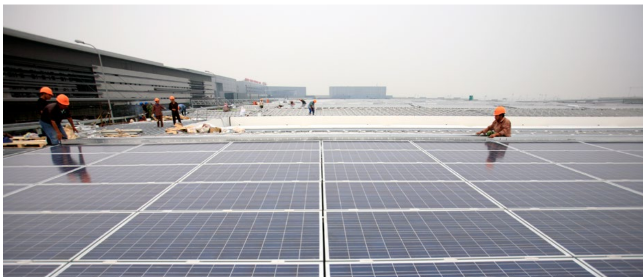
Figure 15: Installation of solar panels on the roof of the Hongqiao Passenger Rail Terminal in Shanghai, China.
