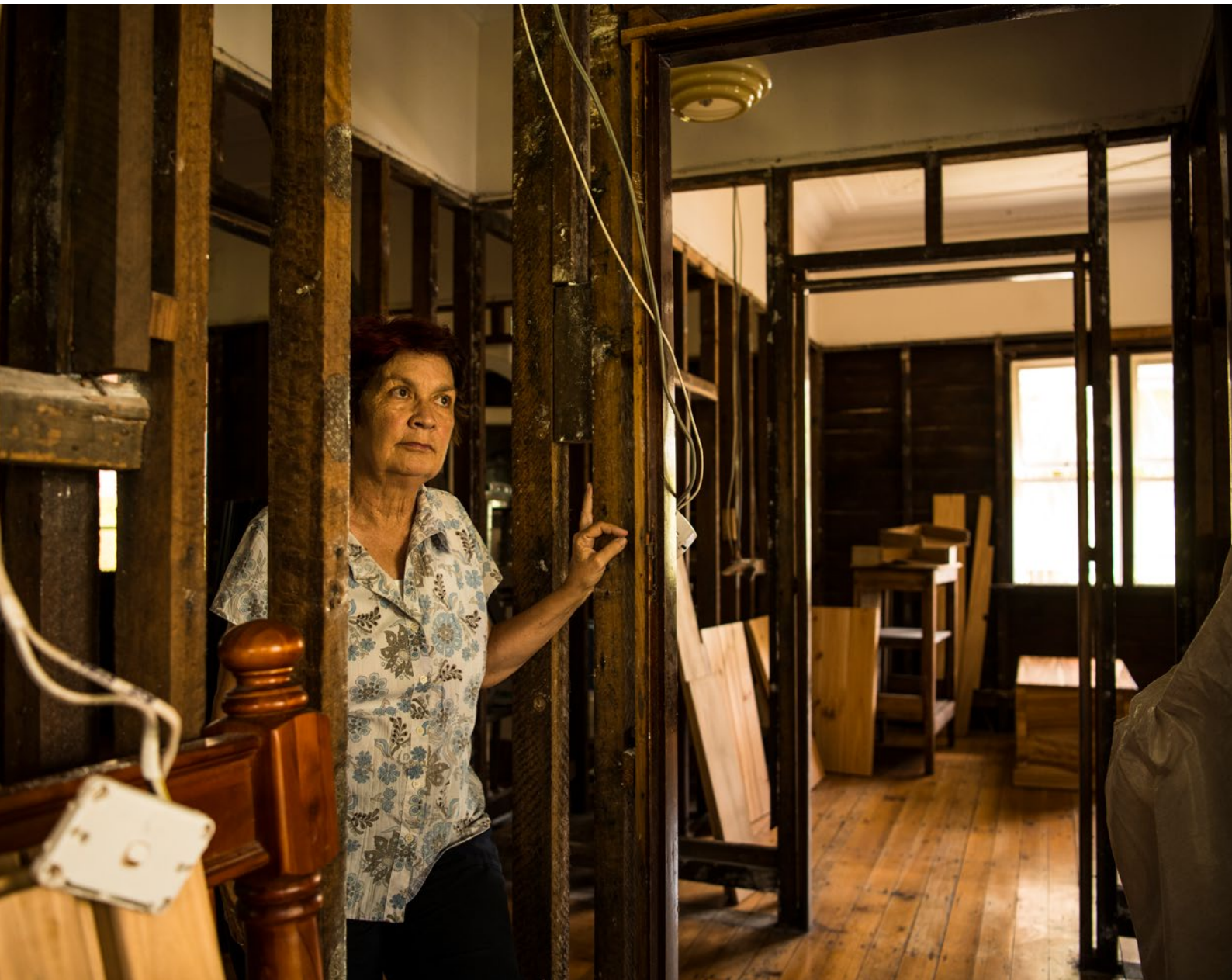
Image 3: Hitting home: Susan Conroy, inside her home in Cathcart Street, East Lismore, nearly one year after the city's worst-ever flood struck in late February, 2022. Floodwaters reached 14.4 metres, two metres higher than the previous record set in 1974.
